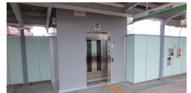
New elevator installed on the Koya Line platform at Kishinosato-Tamade Station
