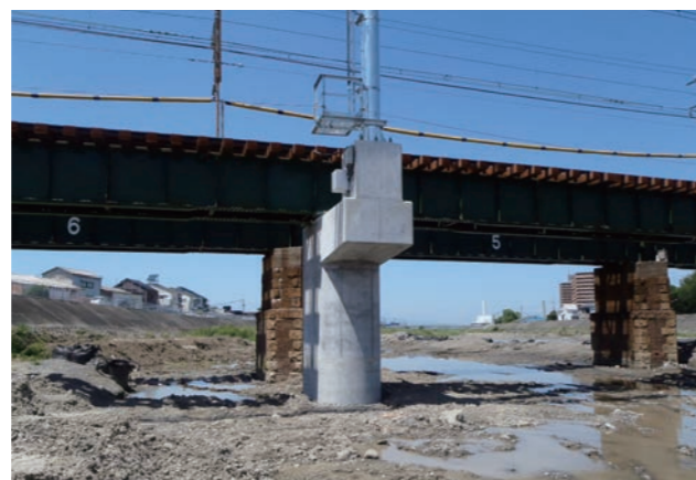
Measuring equipment installed at all 12 bridge pier locations
