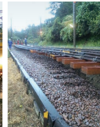
Occurrence of ground erosion
