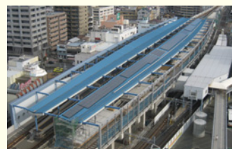
The solar power generation system at Izumiotsu Station
