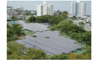
Tannowa Solar Power Plant
