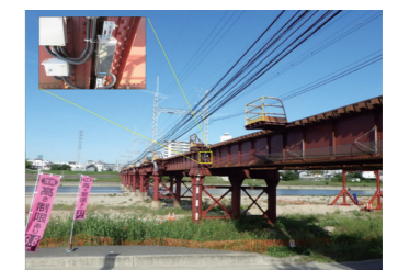
Bridge Abnormality Detection System (Yamato River bridge on the Koya Line)
