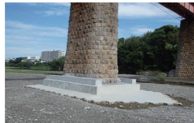
Construction to prevent scouring on the P3 bridge pier at the Kinokawa River Bridge on the Koya Line
