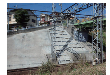
Slope collapse countermeasures (between Chiyoda Station and Kawachinagano Station)
