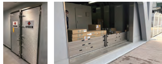
Watertight door (left) and a tide embankment (right) (Tamade General Office)
