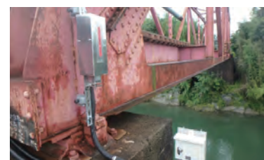
Bridge Abnormality Detection System (Kinokawa River bridge on the Koya Line)
